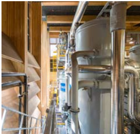
Walkway - Oxidizer to Gasifier
