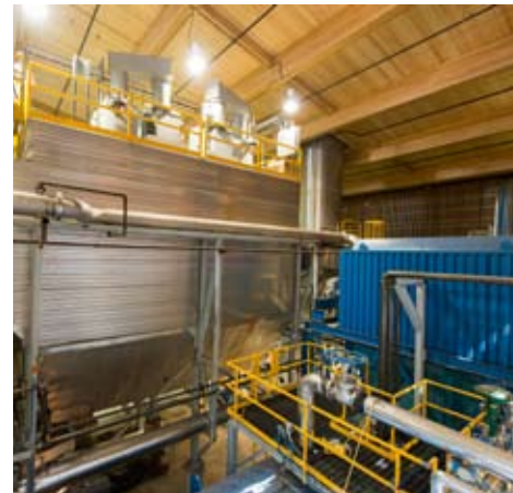
ESP and Boiler
