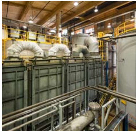
Syngas Thermal Cracking/Conditioning System
