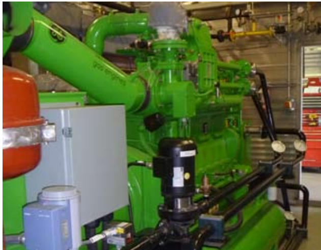
239 kW e Jenbacher Engine at PDC
